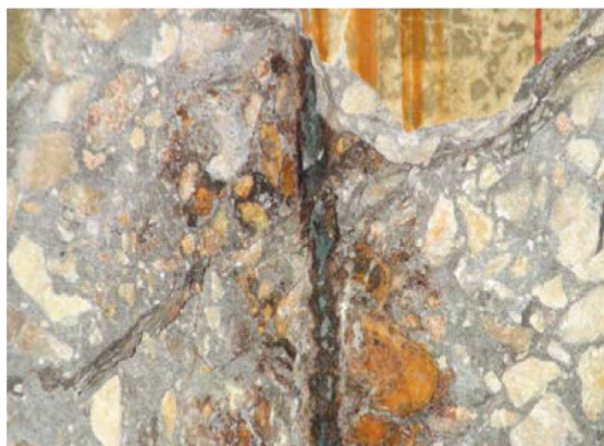
(b) Stirrup rupture failure (30-200-2)
