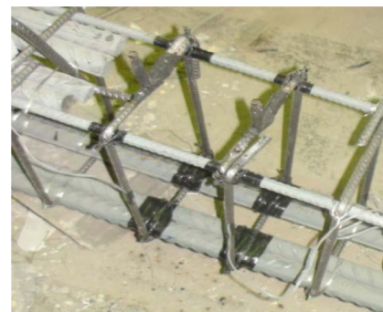
Fig. 2. Stirrup electrical connection
